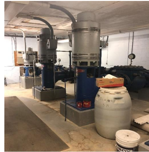
Raw Water Pump Station
